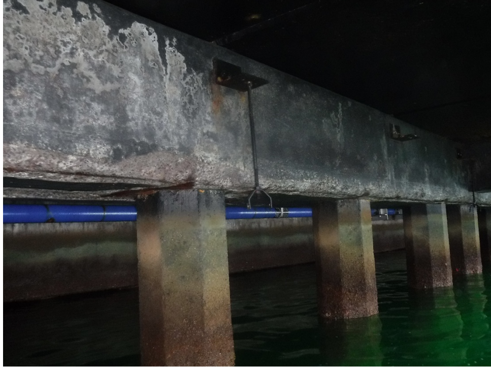
Photo 3: Typical Beam Spall
