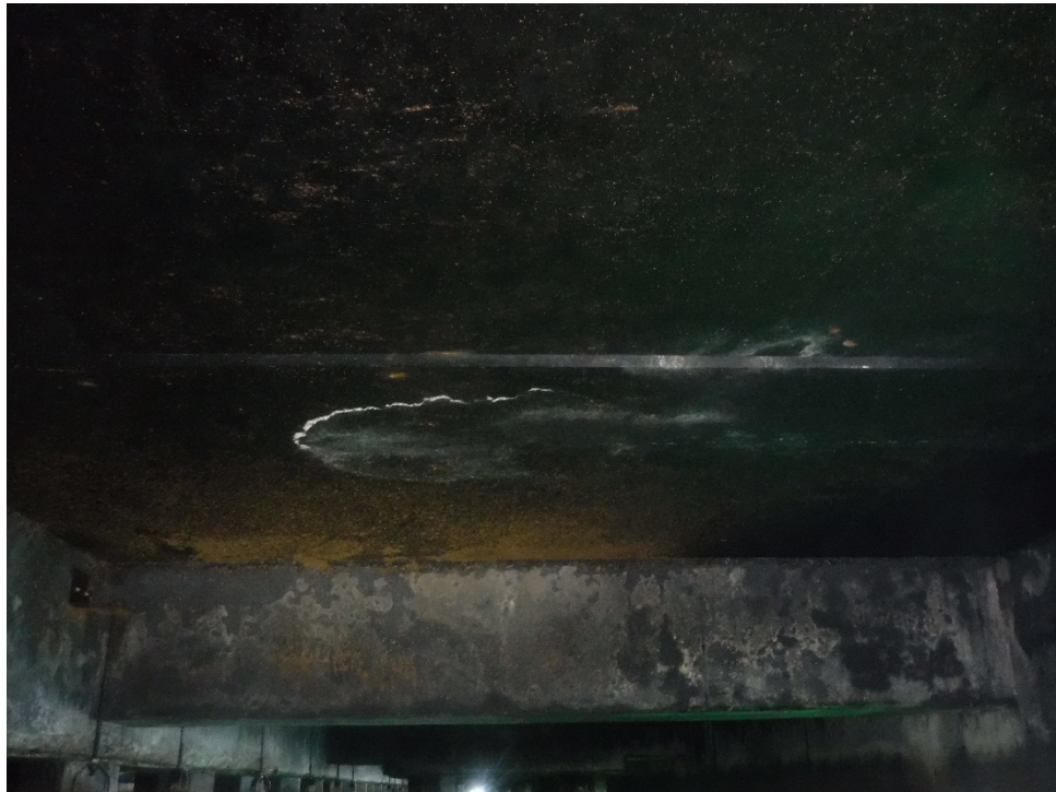
Photo 4: Typical Precast Plank Spall
